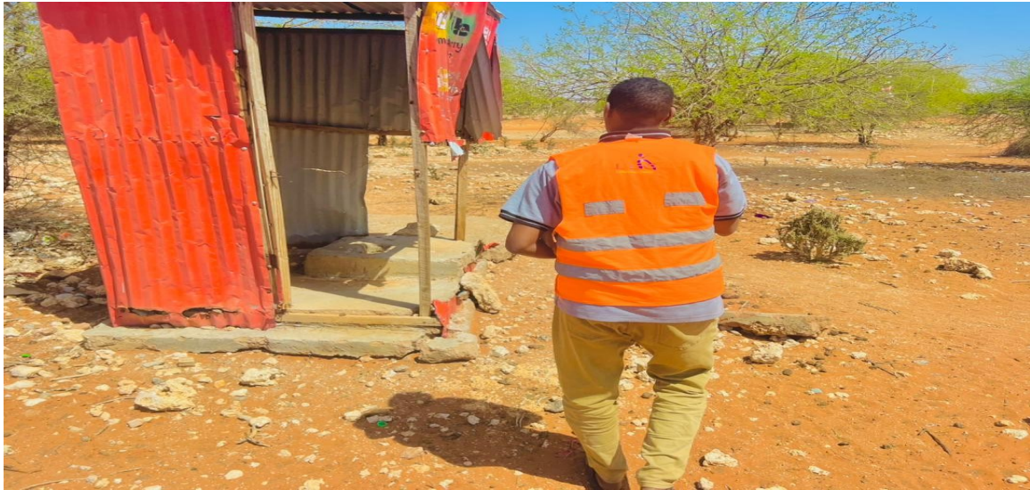
Figure 6: Dilapidated Latrine in Gedo
